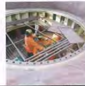
Two workers found without helmet strip at working area
