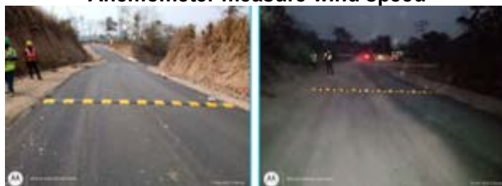
Speed braker installed all road
