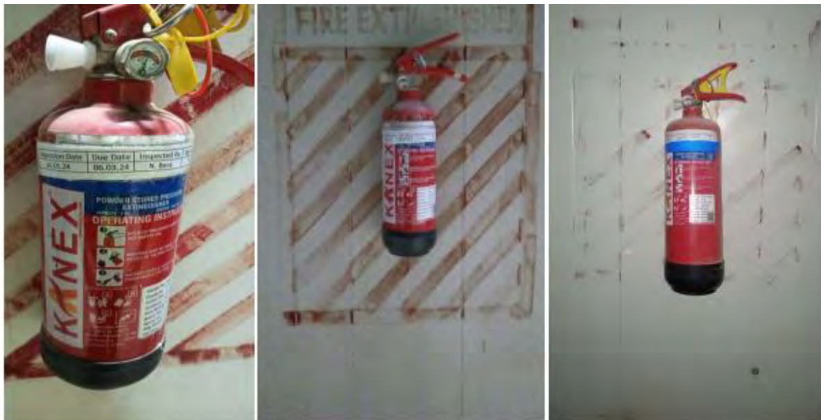
Fire extinguisher inspection CP-2
