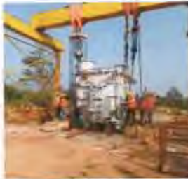
Without estimating the weight while unloading hen the load was lifted the sling were slipped.
