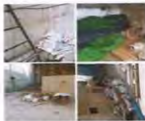
According to supervision fail to maintain house keeping poor housekeeping at working at site.
