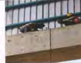
While working at height two workers were seen working without full body harness at height.
