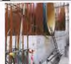
Electrical power supply cable found laying on water and poor insulation on cable joints at U2 DT Cone entrance area.
