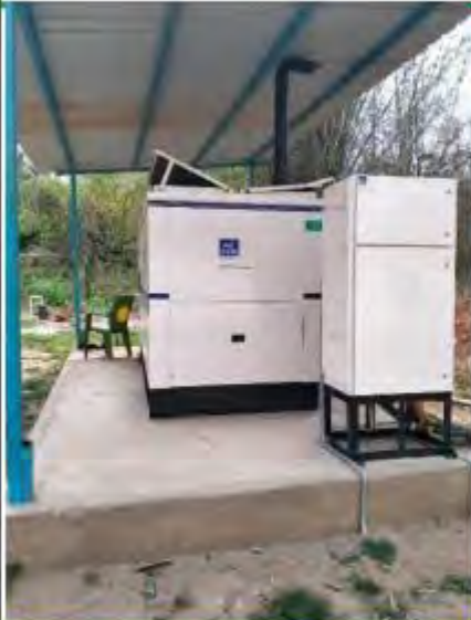
Proper storage area for the DG Set with stack
