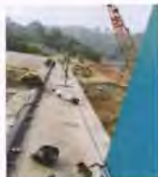
according to supervision without lifeline workers are engaged in job at height of 10 M.
